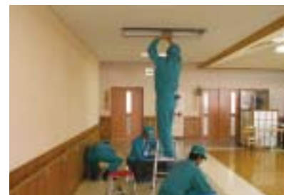
Cleaning electrical equipment at a social welfare facility
