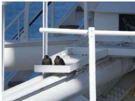
Installed artificial nesting boxes at Shin-Onoda Power Station (Sanyo-Onoda City, Yamaguchi Prefecture) to protect peregrine falcons, a threatened species
