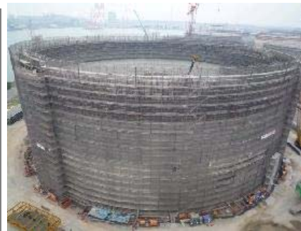
Overview of the construction of the new LNG tank in Mizushima (November,2008)
