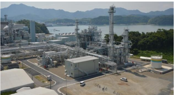
[CO 2 Separation and Recovery Facility]
