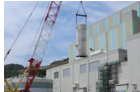
Installation of filtered venting system (Unit 3)
