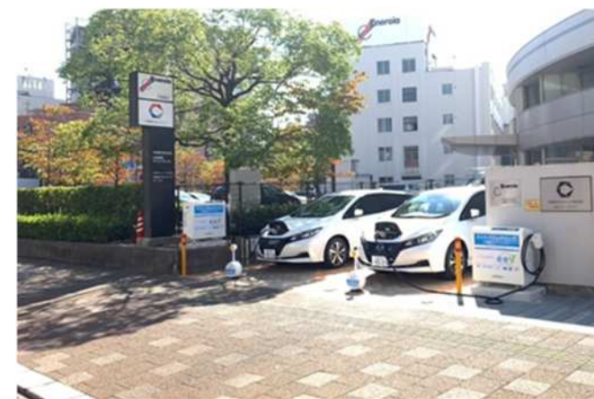
EV charging station at Takeyacho
