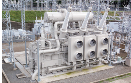
Extra-high voltage transformer (400,000 kVA) at Okayama Substation
