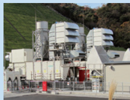
Gas turbine generators
