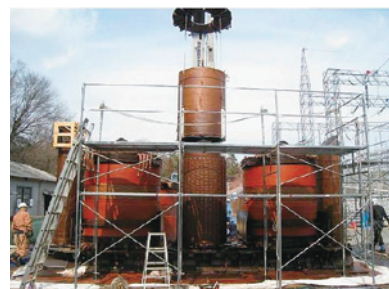
Survey of transformer coil deterioration
