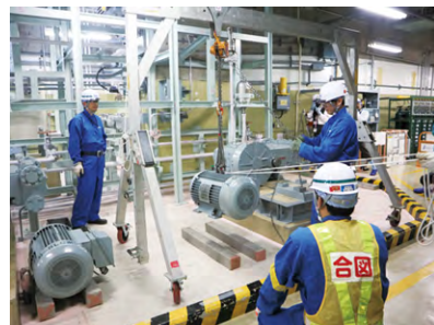
Work to dismantle and dispose of equipment related to toxic liquids (second stage work)
