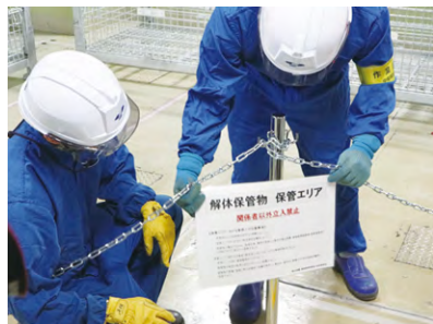
Organizing a temporary storage area for dismantled equipment (second stage preparatory work)
